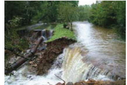
Damage to the city water system in Asheville, North Carolina, due to heavy rain in 2004.
