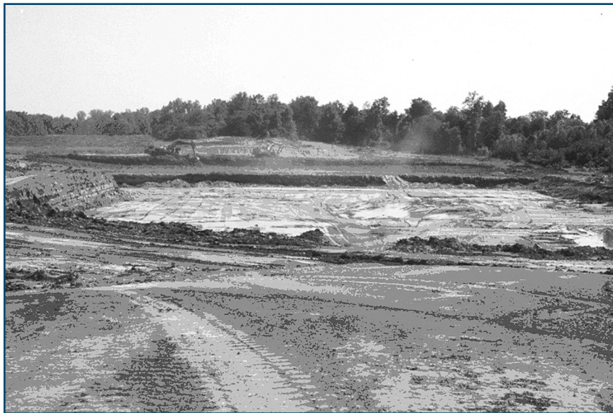
Digging up construction material for the Corps' Mississippi Mainline Levee Enlargement Project in Mississippi. More than 5,450 acres of wetlands will be dug up in this way to construct this flood protection project. Photo courtesy of Melissa Samet.
